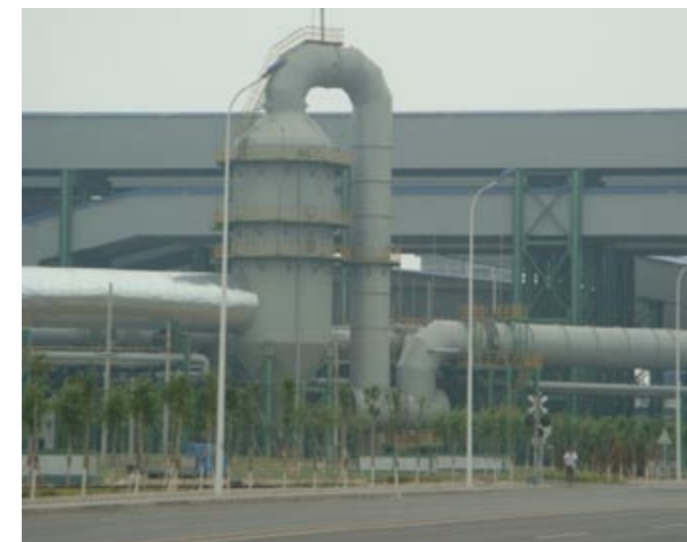
喷碱脱氯防腐装置外景 Exterior view of the anti-corrosive device with alkali sprinkling and dechlorination
