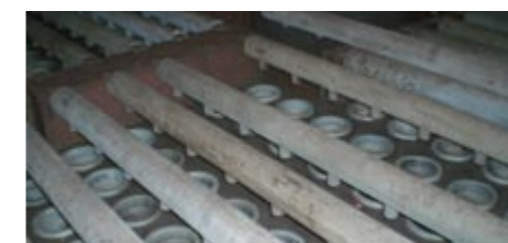
生产中的设备净气箱侧 A view of gas purification box during production
