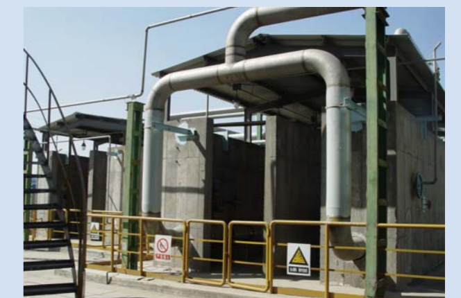
氧气调压站 Oxygen Pressure Regulating Station
