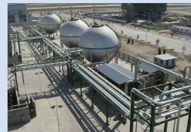
球罐区及管网 Spherical tank Zone and Pipe Network
